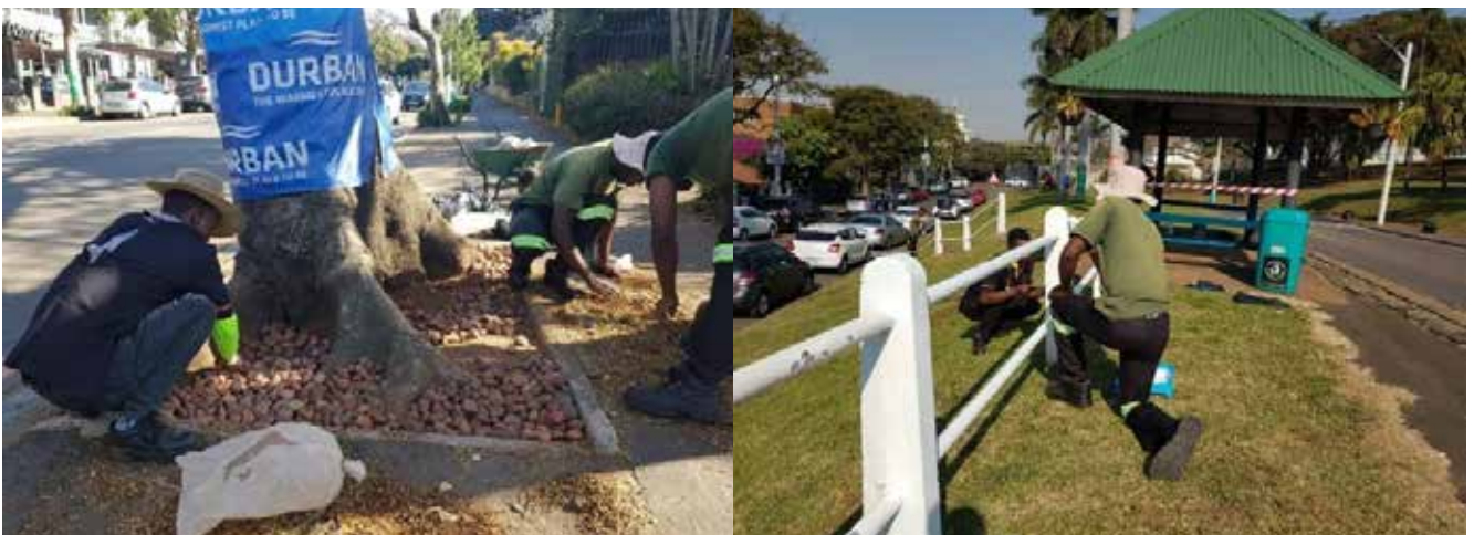
Enthusiastic landscaping division members packing pebbles and painting fences in Florida Road, Durban
